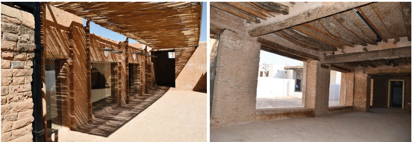
Figure 16. Khalifa House: Restored Shura Court and entrance. Building elements - restored roofs, wall repointing, and the removal of modern insertions. The result is the restoration of the Shura Court, the rediscovery of the historic veranda where the Khalifa held court.
