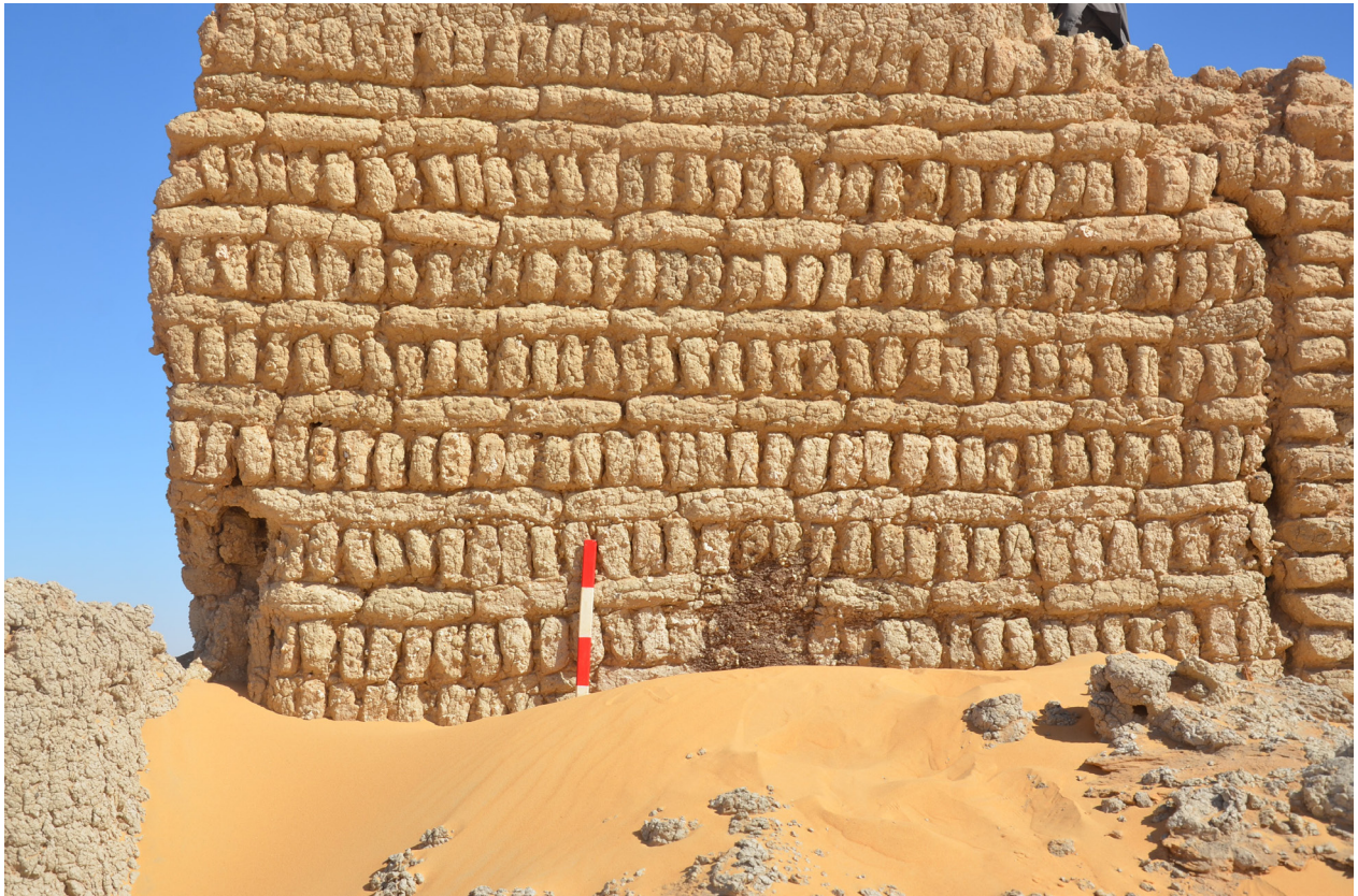
Figure 7. Detailed view of the wall structures views from the tower walls (photograph by Hamad Hamdeen).
