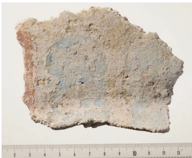
Figure 7. Fragment of render on a cornice coated with limestone wash (Phase 3).
