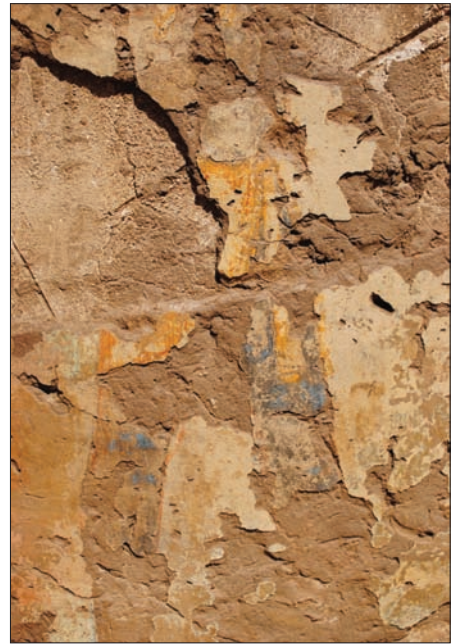
Plate 5. Column with a layer of mud plaster overtop of a lime plaster scratch coat. Lime wash and pigments have been applied to the mud plaster.
