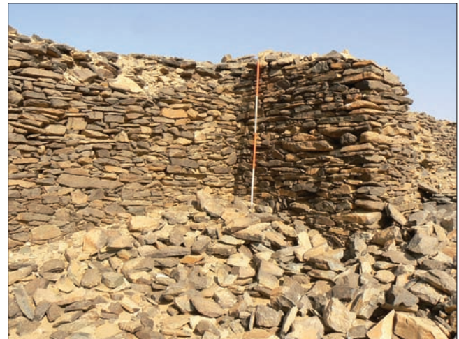
Plate 2. Site AS 1 – junction of the eastern projecting tower with the enclosure wall (photo. M. Drzewiecki).
